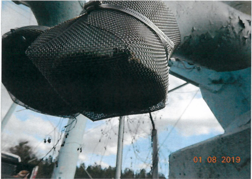
Overflow Pipe Picture
