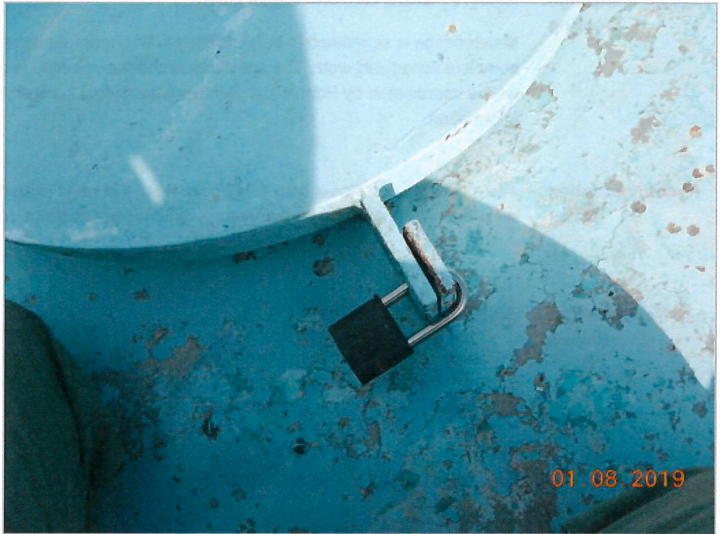
Access Hatch Picture
